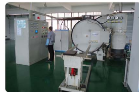
Vacuum brazing furnace
